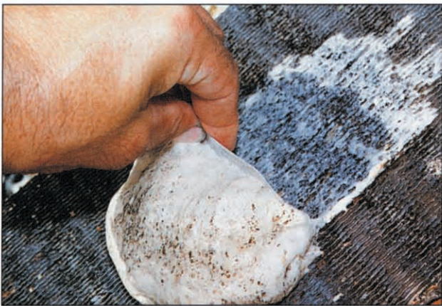
If properly maintained and regularly cleaned with coil cleaners and hot water, a coil's interior as well as its exterior can be kept clean. The bubbling action of foaming cleaners can actually lift the dirt from the coil's interior.
